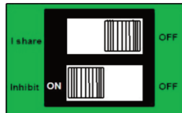
DIP Switch for Current Share & Inhibit/Enable for powerMods XgG to XgL and Xg1 to Xg5
