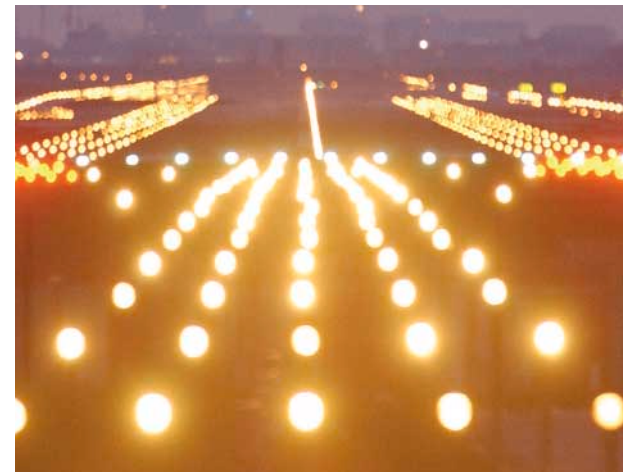
RUNWAY LIGHTING - HALOGEN
