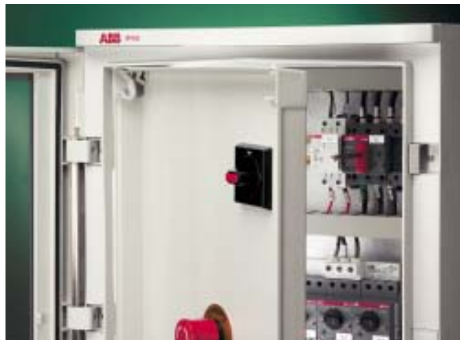
Example of the configuration of a switchboard for an automation application: some ABB control and protection devices are installed on the plate. The inner door is fitted with light-signaling devices.
