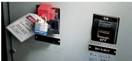
Oversized Breaker Lockout Device
