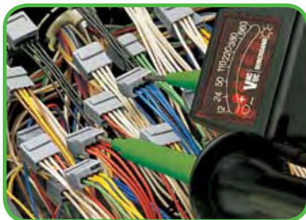
Test using integrated test ports
