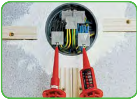
Voltage testing of push-wire connectors
