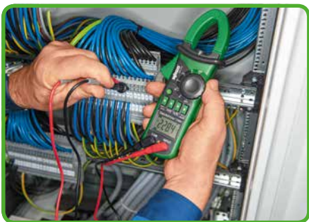
Voltage testing in switchgear cabinet
