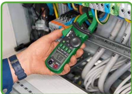
Current measurement in switchgear cabinet
