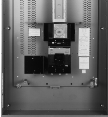
Main Circuit Breaker and Solid Neutral Compartment (Canada service entrance not shown)
