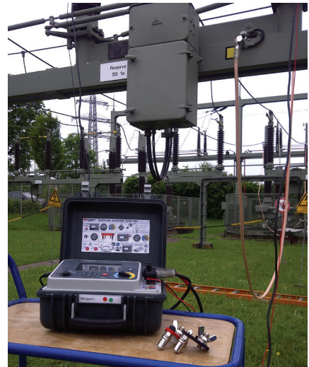
DLRO100 testing circuit breaker
