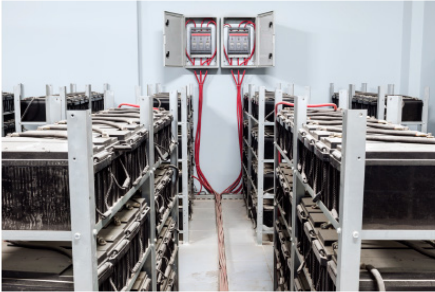
Figure 12a. An example of a battery storage room and Keysight instruments for electrical maintenance measurement activities
