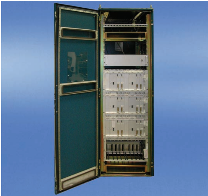
Application: Control system
