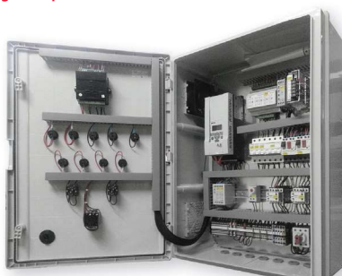
Example of control equipment and accessories installation
