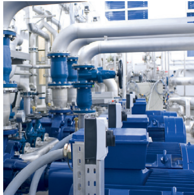
The Ethernet interface enables events-driven transmission of diagnostic information. So, for example, measurement data about the pumps, which is continuously collected throughout their service life, provides information about their performance and operational status.
