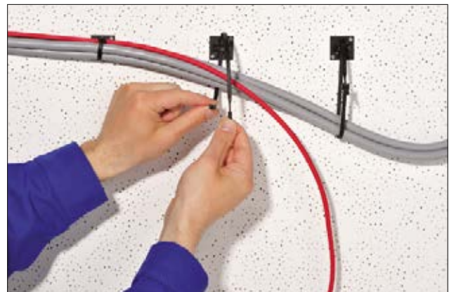
Without additional effort only Q-ties can be used for temporary and final cable bundling.
