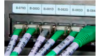
Patch Panel Labels
