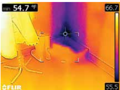
Area box with Cold Spot demonstrates air infiltration
