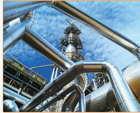
Chemical, Oil and Gas
