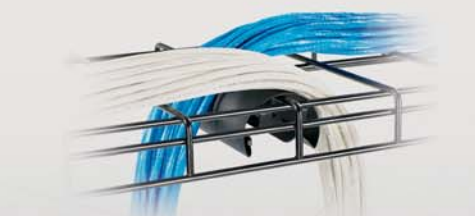
Route redundant ("A" and "B") cabling into adjacent cabinets with a single waterfall.
