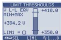
Control and diagnostic
