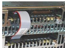
Shelf-to-shelf cable connection (part # CC848848952)
