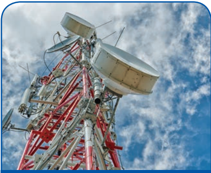
Telecom -Data Infrastructure
