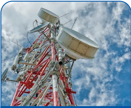
Telecom -Data Infrastructure
