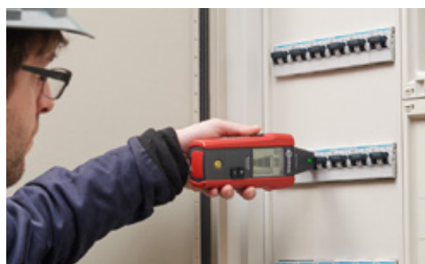
Identify the single correct breaker
