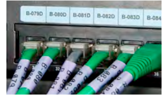
Patch Panel Labels
