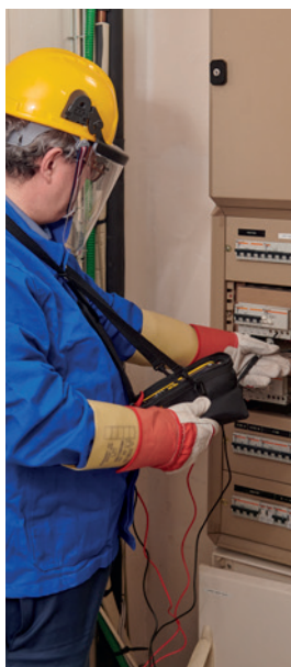
Control of an electrical cabinet
