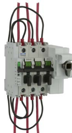
CCP2-PLC-IND fuse monitor mounted on a right front rotary operated switch.
