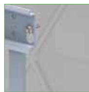
large space for cables
