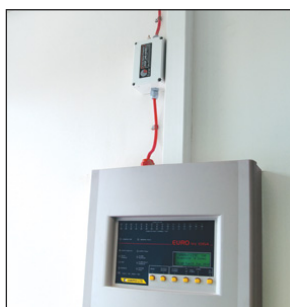
Ready boxed protector (here an ESP 240-5A/BX) installed on the fused connection (spur) to an alarm panel
