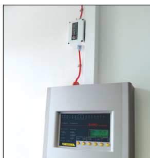
Ready boxed protector (here an ESP 240-5A/BX) installed on the fused connection (spur) to an alarm panel
