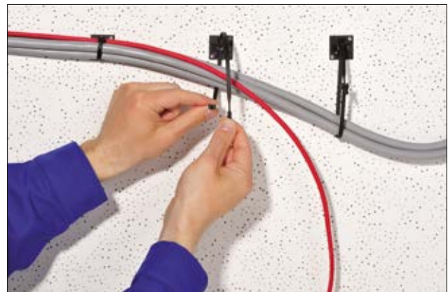
Without additional effort only Q-ties can be used for temporary and final cable bundling.
