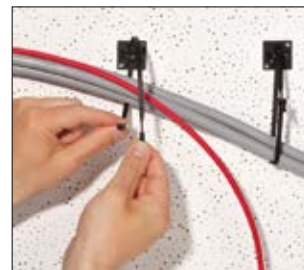
Without additional effort only Q-ties can be used for temporary and final cable bundling.
