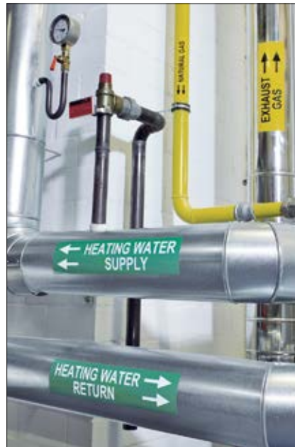
Large and highly visible pipe marking.
