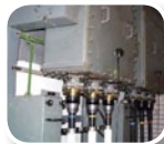
Power sensitive equipment
