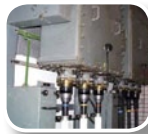
Power sensitive equipment
