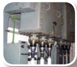
Power sensitive equipment
