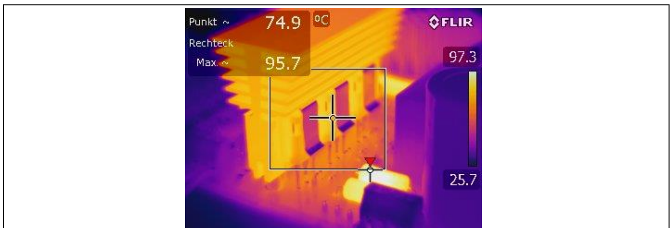
Figure 31 Thermal image of right power MOSFETs (hotspot at the capacitor's balancing resistors)
