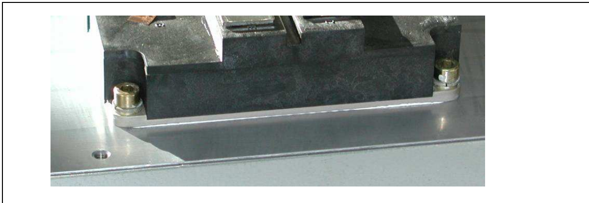
Fig. 9: Module edges show leaking of excessive paste
