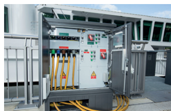
Dock power distribution systems
