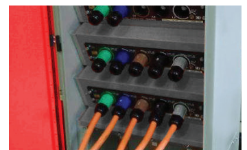
Emergency power systems
