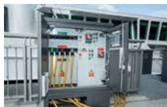
Dock power distribution systems
