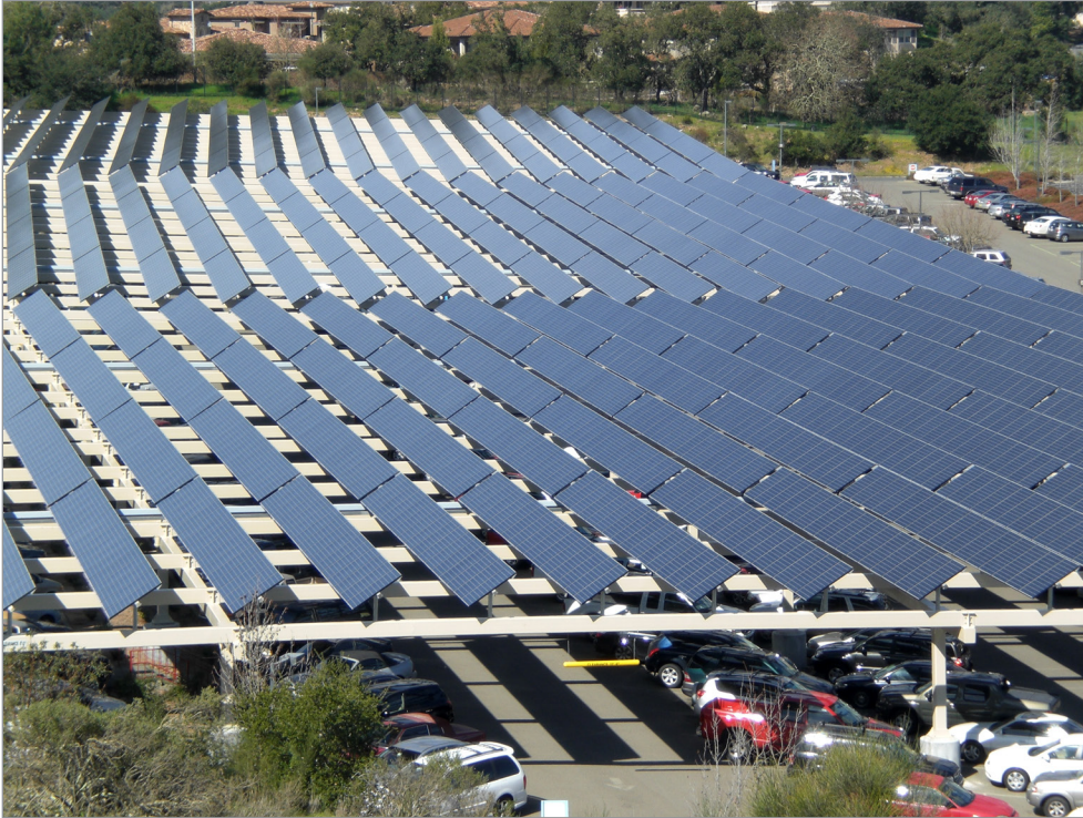
Figure 1. Solar panels at the carpark of Keysight Technologies, Santa Rosa, CA.
