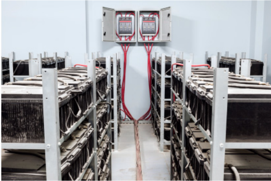
Figure 12a. An example of a battery storage room and Keysight instruments for electrical maintenance measurement activities
