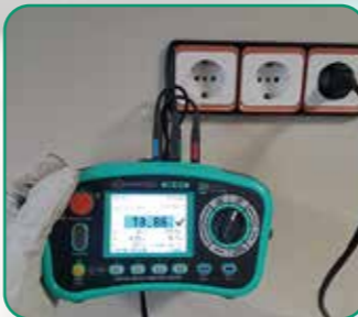
Loop test from a wall socket
