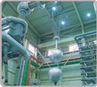
High Voltage Test / Impulse Test
