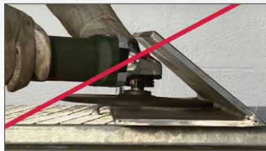
This solution violates safety standards
