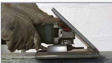
Typical problem...Grinder doesn't reach
