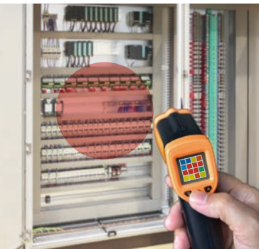
Transformers & distribution boards
