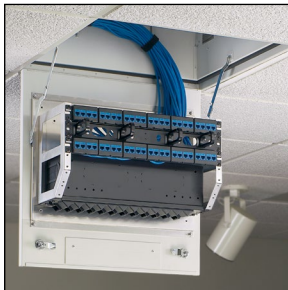
Zone Cable Boxes
