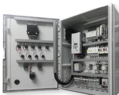
Example of control equipment and accessories installation
