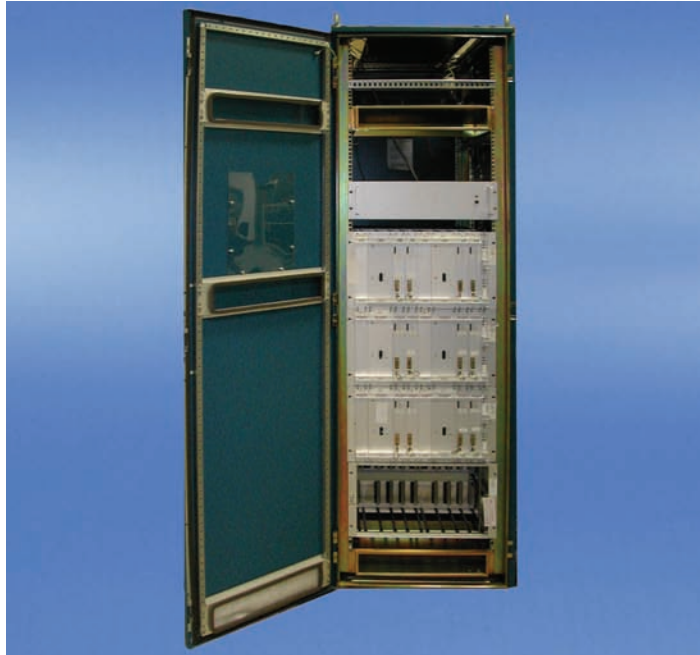
Application: Control system Csee_DSCN2296
