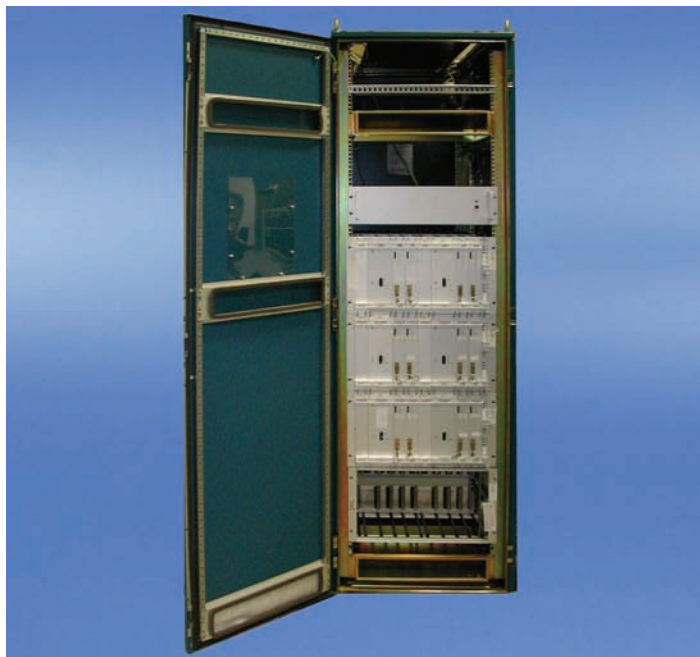
Application: Control system Csee_DSCN2296
