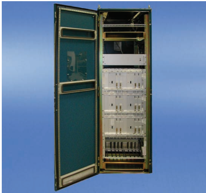
Application: Control system Csee_DSCN2296
