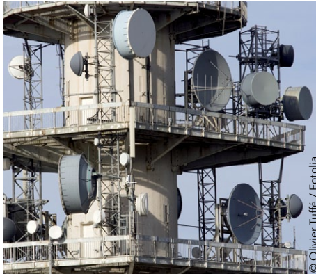
Telecom - Data infrastructure
