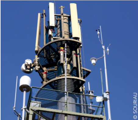
Fiber to the Antenna
